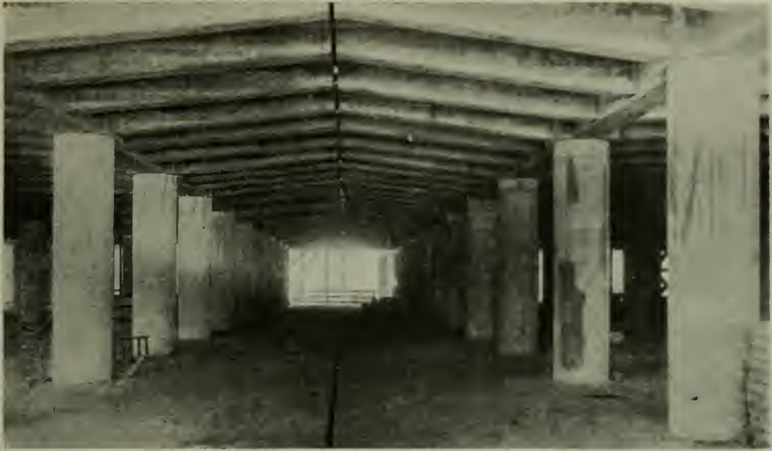
REINFORCED CONCRETE BOTTLING BUILDING, ST. LOUIS : TYPICAL INTERIOR VIEW, SHOWING EXPANSION JOINTS.
